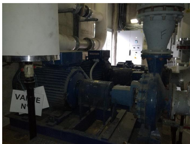
Figure 9. Pompes de circulation Figure 10.
